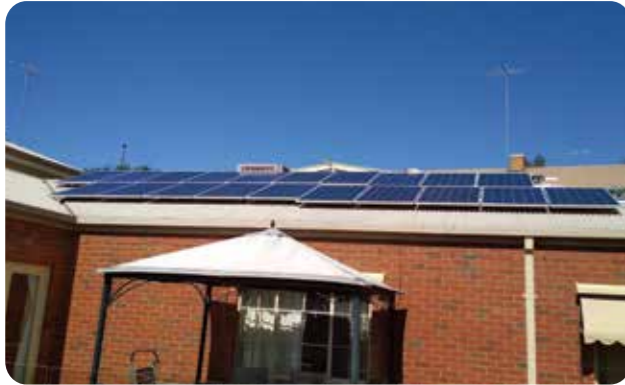
Location: Melbourne, Australia Capacity: 6KW Model: MG6KTL
