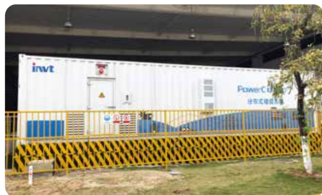
Location: Guangdong,China Capacity: 500kW/1.8MWh Model: BD500KTR-T
